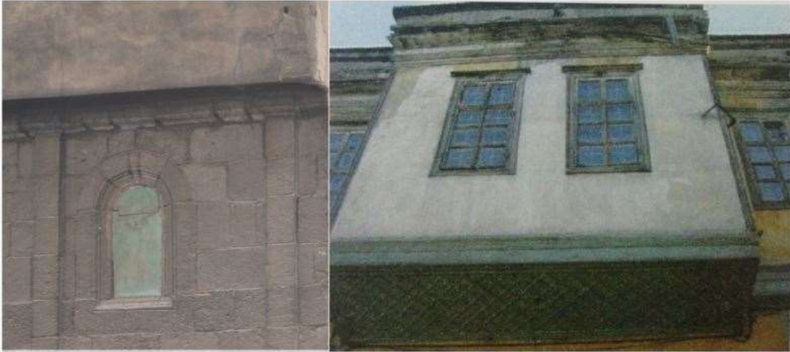
Fig. 5. Ground floor made of cut stone and first floor covered with plaster
