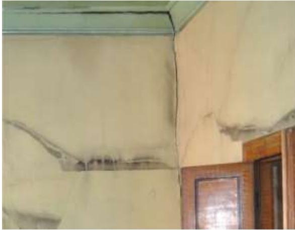
Fig. 7. Deep structural crack in the walls
