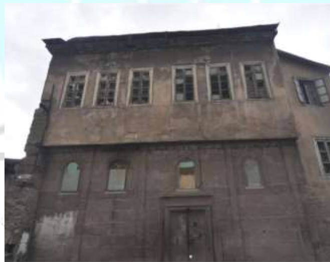
Fig. 6. Plaster spills and joint gaps observed on the second floor of the building
