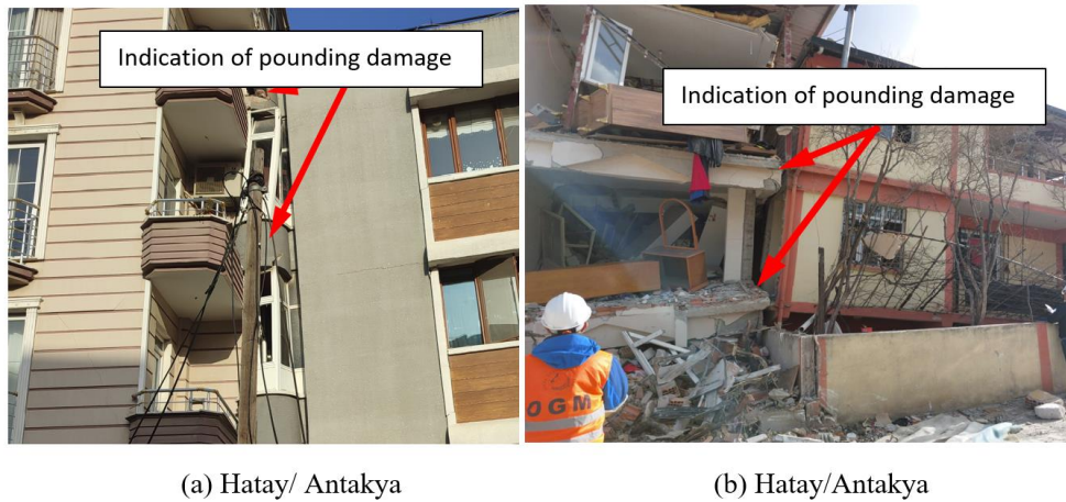
Figure 6. Damages related to inadequate distances between neighbouring structures
